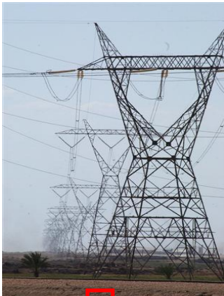
High Voltage Utility Distribution
