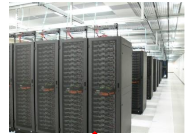
IT Load (servers, storage, Net, ...)
